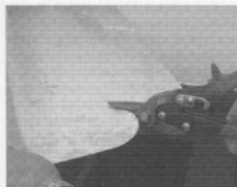
Figure 3. Using right hand tin snips to cut the rotor disks from a sheet of 20 gage type 304 stainless steel.
